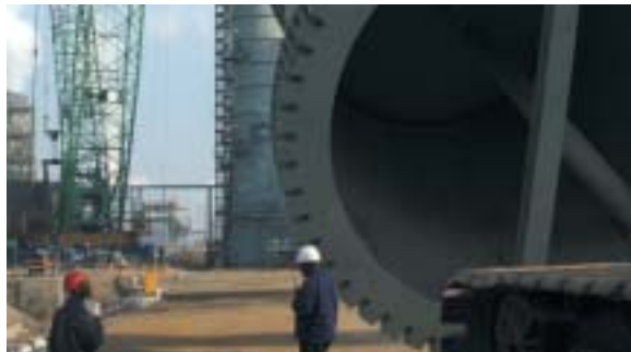
A 550 t distillation column being erected for the second 1-octene train at Secunda.
